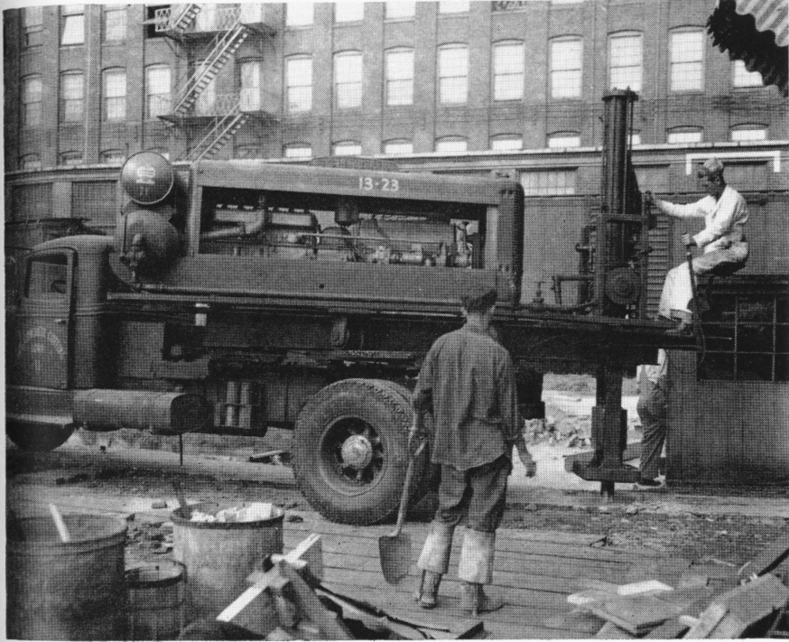
This more or less innocent looking vehicle which is being used to break up the old foundations of Scovill's streets packs a tremendous wallop in its rear end. It breaks up the concrete so's the steam shovel can get it.
